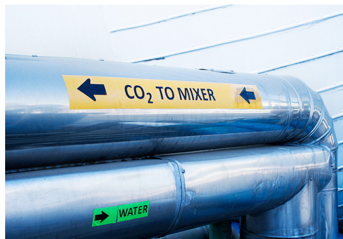
Figure 3-3. CO 2 pipeline infrastructure will be decisive for enabling carbon capture for blue ammonia production.
