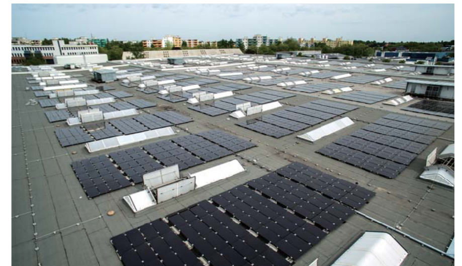
Hybrid power plant at GE Power Conversion production site in Berlin
